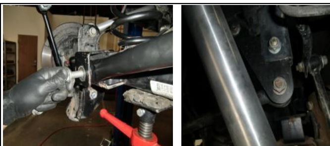
27. Install the new track bar into the frame pocket and axle mount.
