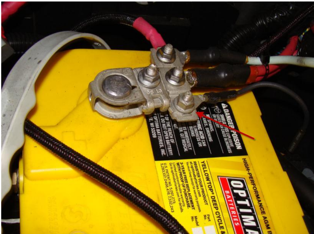
Figure 6 – Black 20g POSITIVE wire connected to POSITIVE battery terminal
